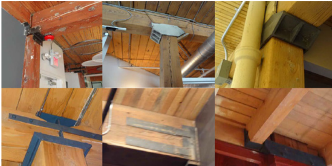
Figure 2.2. Typical historic post and beam connections (from Appendix C-2, Koo, 2013). Metal castings provide end-grain bearing to reduce the effects of wood shrinkage.
