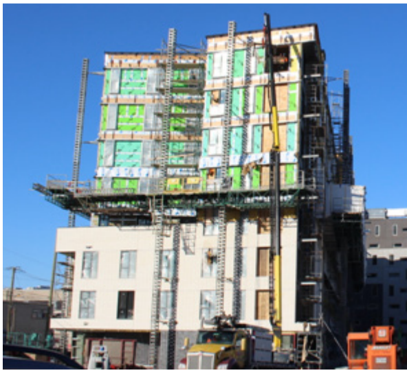
Figure 2.15. Arbora, Montreal. 8-storeys, first of three buildings on this site. (Photo D. Moses)
