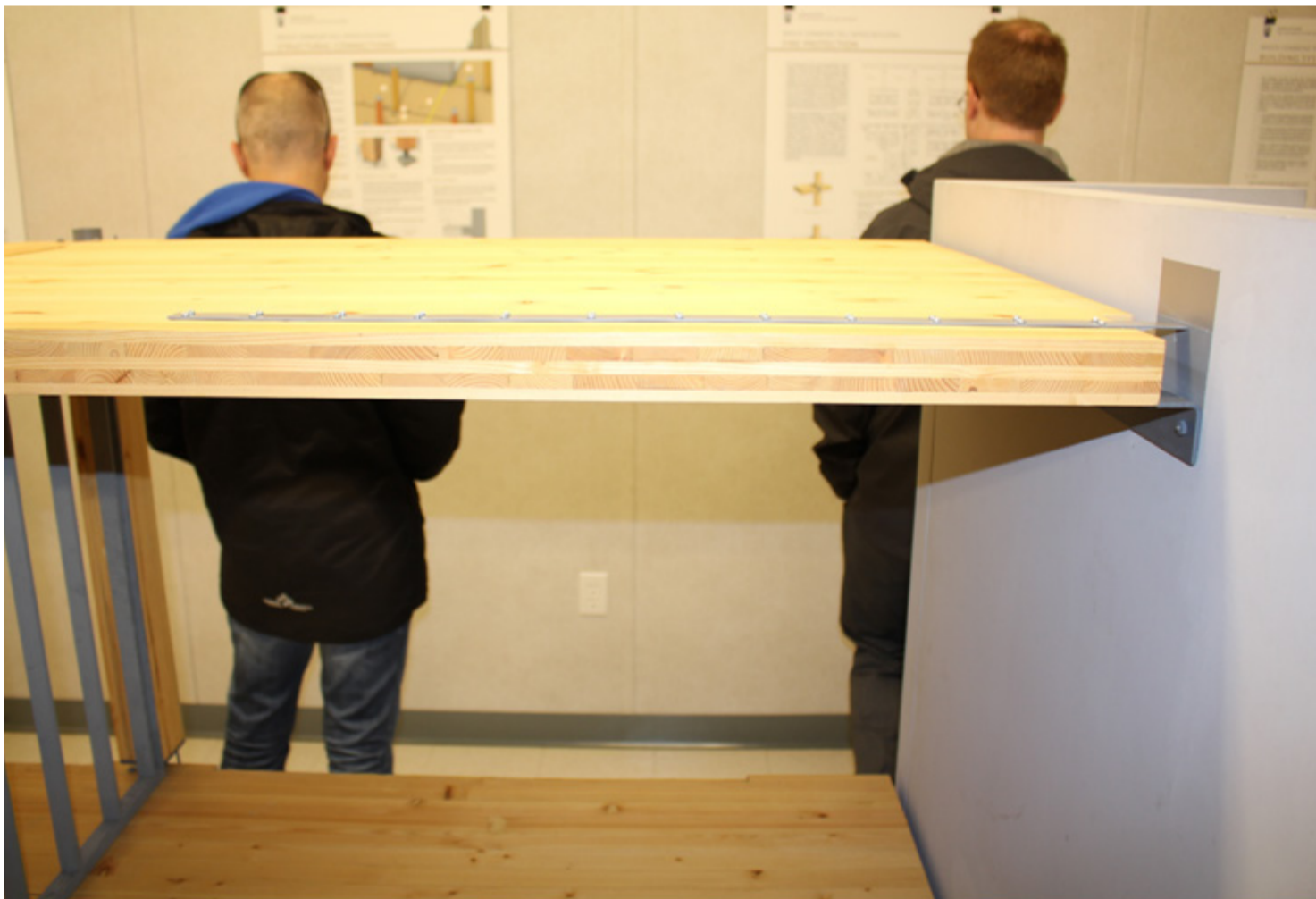
Figure 4.7. UBC Brock Commons demonstration connection of a CLT panel to concrete shear wall with tension strap and vertically slotted connection (Photo: D. Moses)
